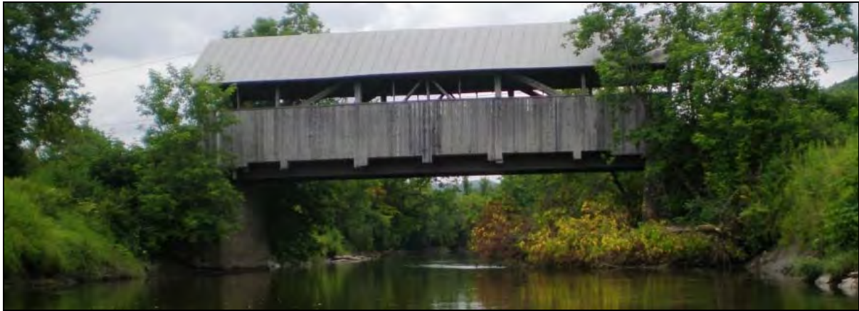
Figure 12: The Coburn Covered bridge (R24) was elevated to increase the area through which water can flow. Despite this, the bridge abutments still constrict the channel and upstream and downstream erosion is a result (see fallen tree on right bank).
