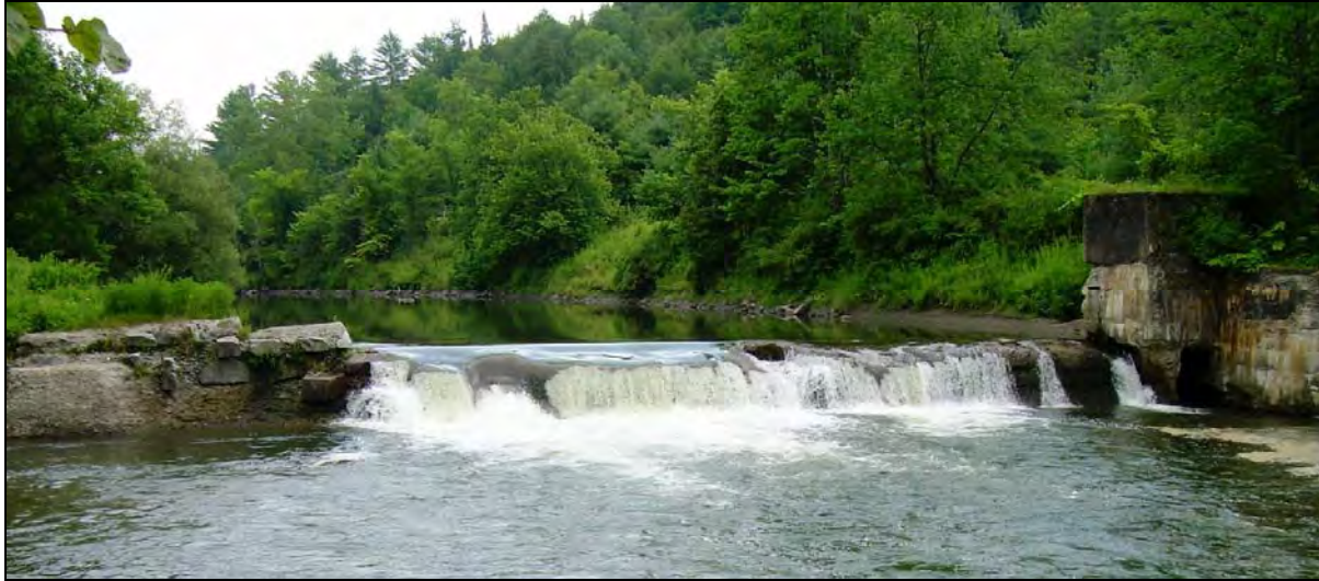
Figure 15: An old concrete dam disrupts water and sediment transport at reach R21-A (looking upstream).
