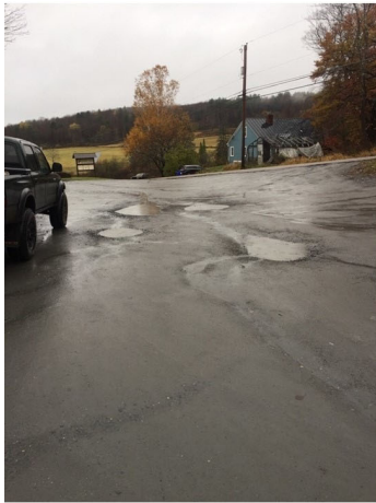
Puddles and potholes in the upper parking lot.
