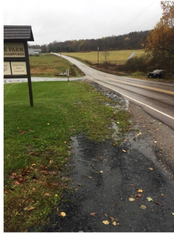
Drainage from the upper parking lot and County Rd flows along the grass and over the lower driveway.
